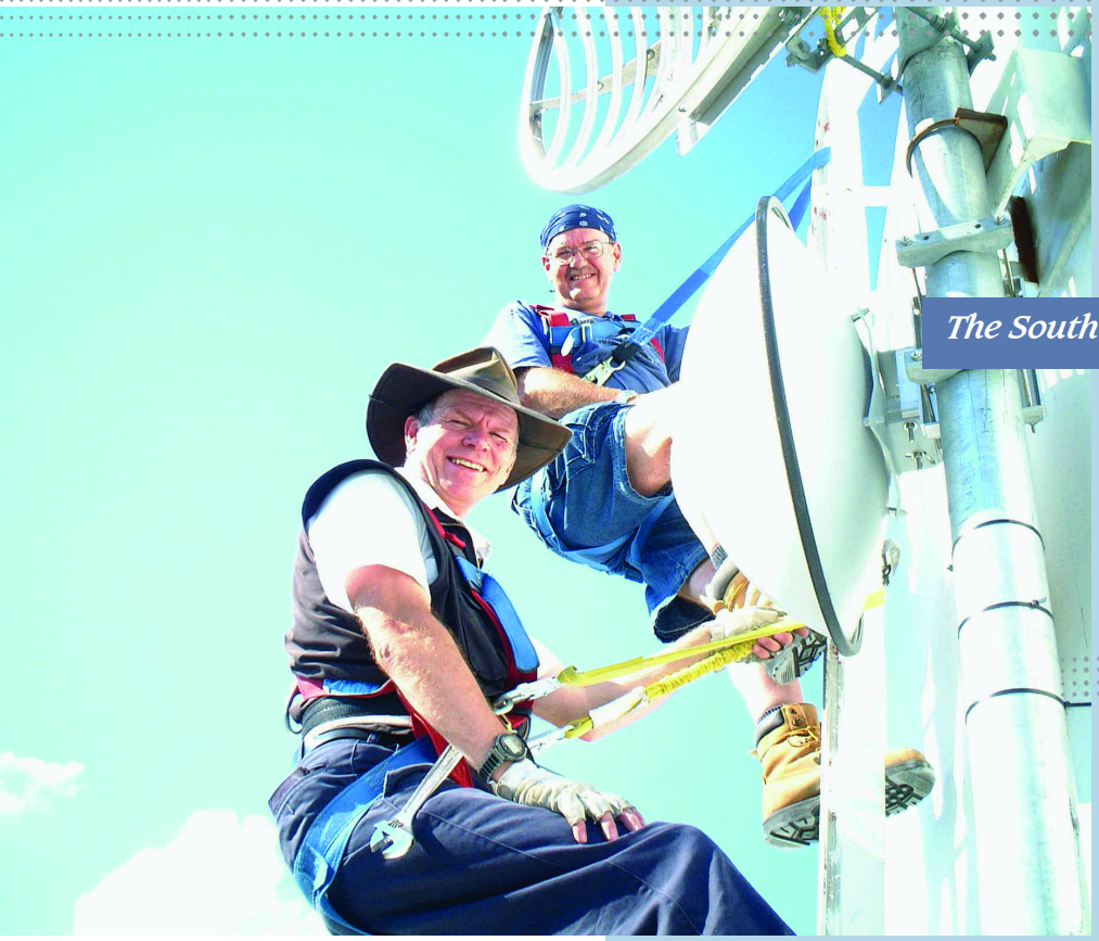
Roy Brister and Max Tom install wireless equipment on the Cardinal water tower. Taking fate into their own hands, South Dundas has proven that bandwidth equals jobs ... at least in their Ontario East community.
